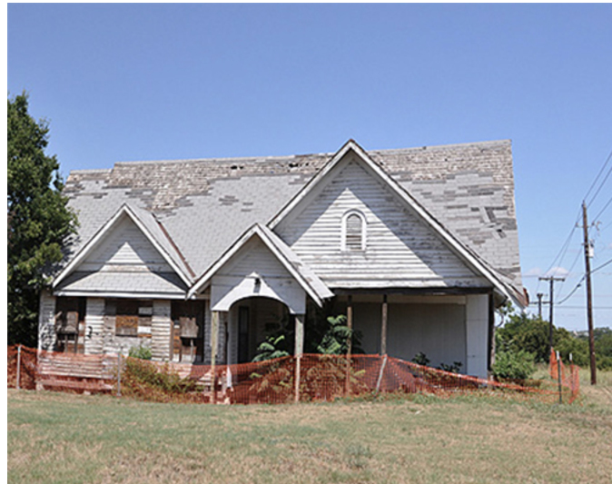
The Dickey House is shown in 1997, before renovations began. Photograph courtesy of Preservation Texas.
