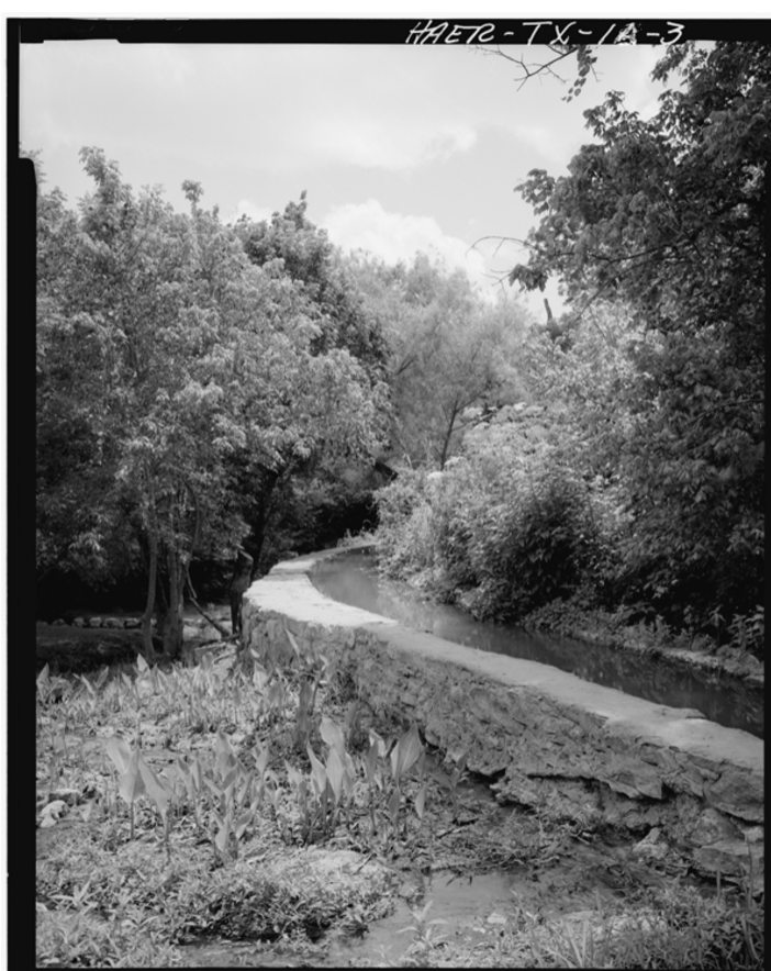
Espada Acequia, Piedras Creek Aqueduct, Spanning Piedras Creek east of Espada Road, San Antonio, Bexar County, Texas. Historic American Engineering Record (Library of Congress).
